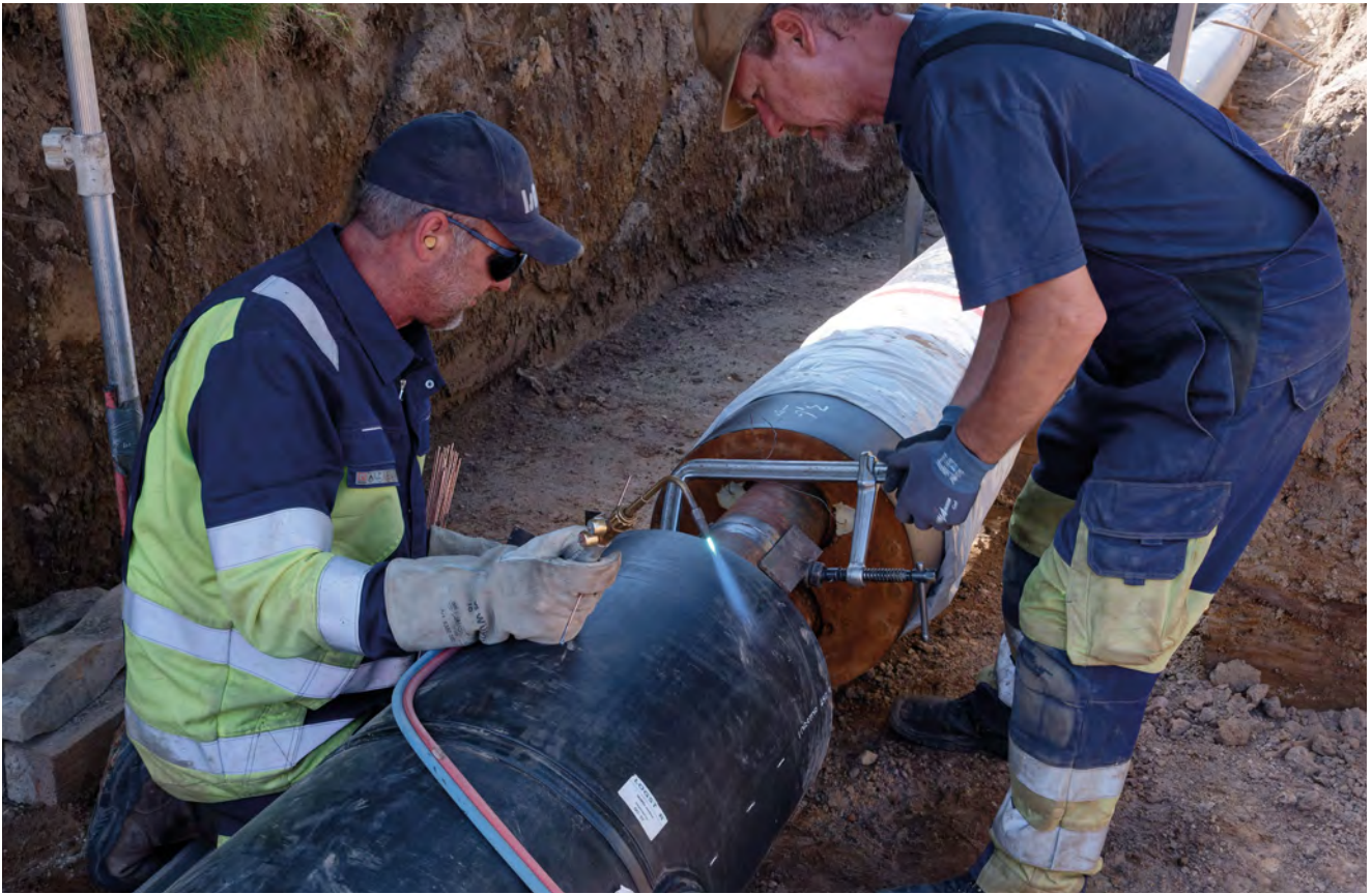
Schleswig-Holstein, Germany, 2023: Laying pipes for a local heating network in Hürup Photo: Stephan Röhl
