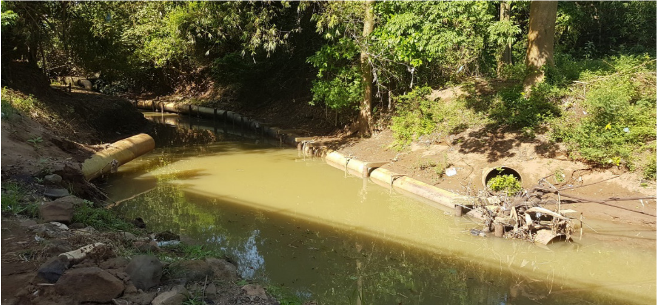
PT RUM direct waste pipe inside Bengawan Solo River during Dry Season, 14 May 2023. (Photo source: Dewi Candraningrum.)
